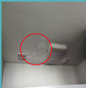
Building in Orange County With Signs of Water Intrusion
