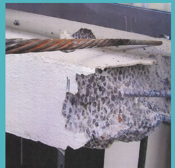
Building in Pinellas County With Corroded Deterioration of Structural Elements
